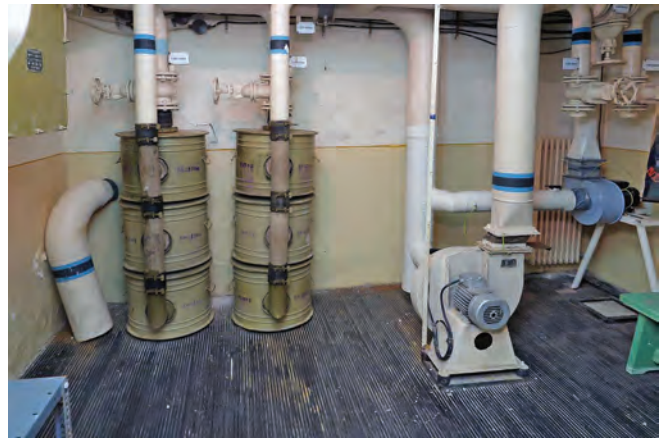
Filter banks and air-handling equipment in the Csepel Control Centre. No evidence of manual operation in the event of power failure
